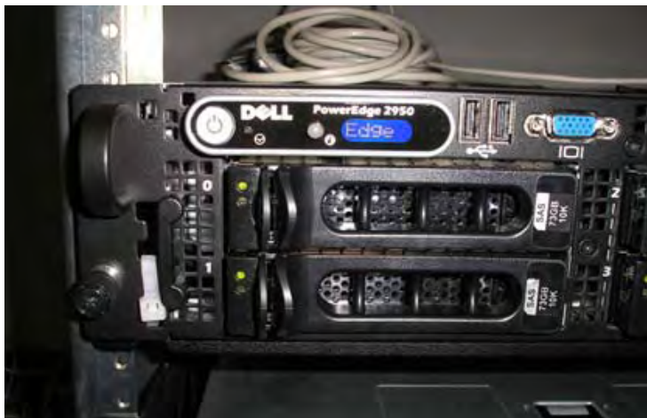
Figure 4. VOD 125/300W (Dell 2950 – Front View)
